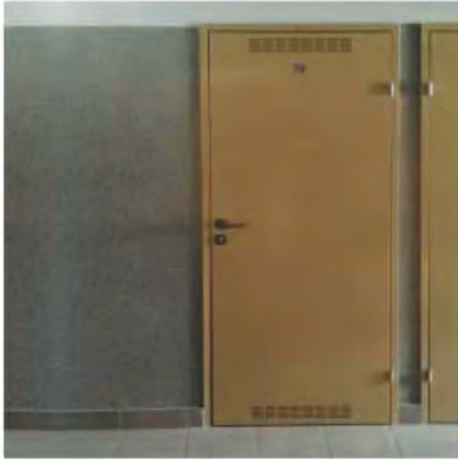
RESIDENTIAL ESTATE UNIVERSAL DOORS TO UTILITY ROOMS
